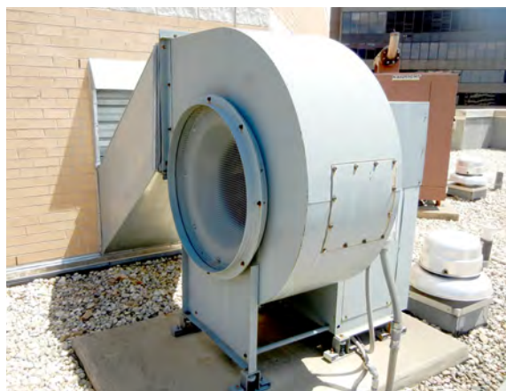
Figure 12.12. A stair pressurization fan.
