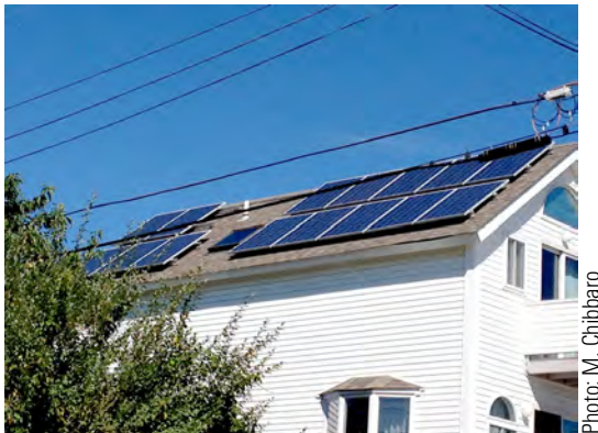
Figure 7.14. Photovoltaic panels on a roof.
